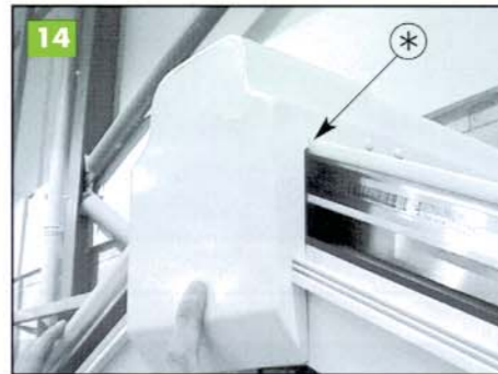
Fit the gable ridge end cap as per the victorian installation guide (ie to suit frame thickness see page 26).
