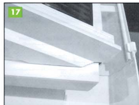
If using 5 & 6 series glazing bars, it is necessary to trim back the fixing bars on the lean to cloaking trim, to allow a flush fit across the face of the gable infill wedge. Fit the lean to cloaking trim.
